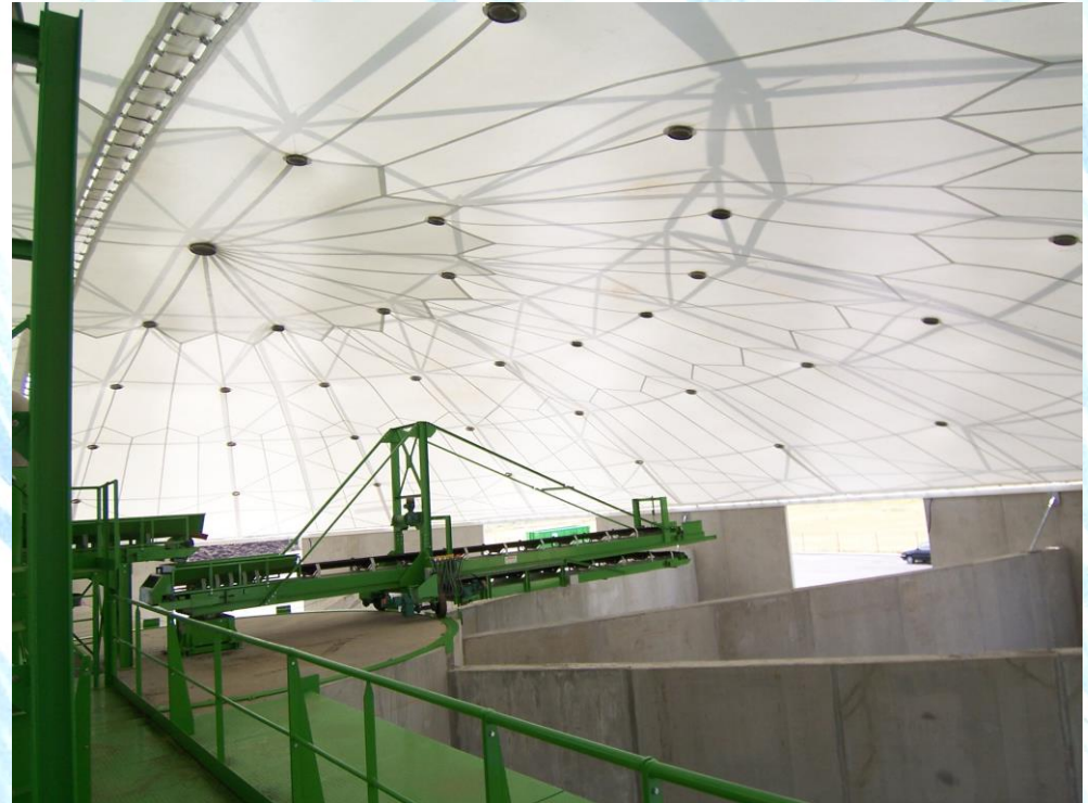
Saint-Eloi - Cugnaux, la Saudrune : Sewage processing center covered with a textile roof
